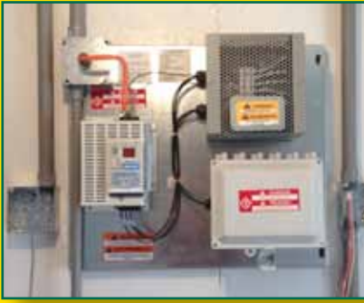
VFD Controls for variable speed operation
