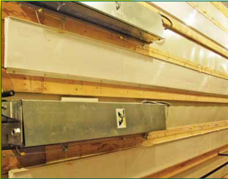
Continuous inlets are designed to run the entire length of the house.
